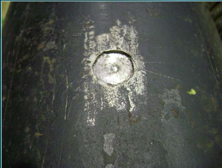
Defect before cladding
