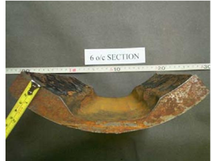
Channelling corrosion in Strathspey W.I. pipeline which was operated under similar conditions
